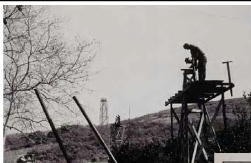
Crossing ravines on stands to keep line horizontal. Pasadena Base measurement. Base line party of Clement L. Garner, 1922
